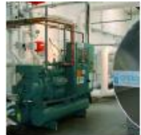
Chiller. Source: Cristopia.
